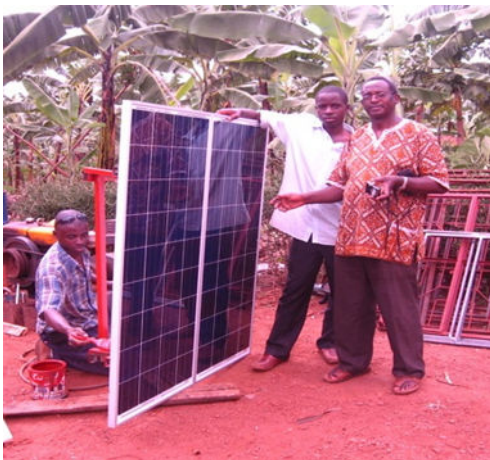
Fr. Ben and workers installing solar panels for lighting at Sacred Heart Girls' Hostel
