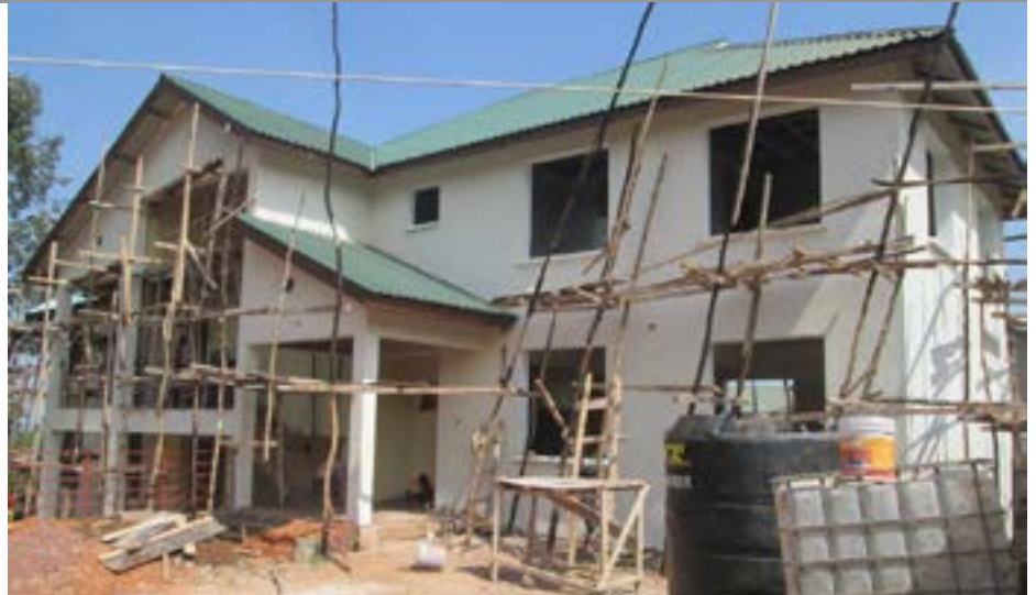
Construction of the kindergarten classroom at St. George Cathedral is well under way!
