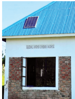
Solar Panel for a girls' dormitory
