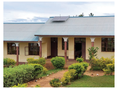
Solar panels on a classroom building
